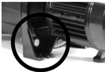
Regularly check the waterproofness! (A leak through a mechanical seal can cause important damages!)
